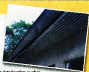
Sagging roofs can be due to deterioration or when lightweight materials are replaced with heavier ones.
