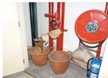
Rubbish at the Bomba riser. Is the fire extinguisher, fire hose inspected for expiry of use?
