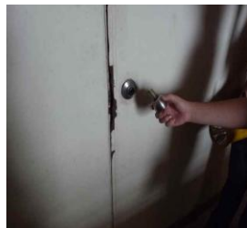
Electrical riser door lock broken - does not comply with 2 Hour Fire rated doorset specifications
