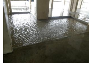
Flooding in covered car-park
