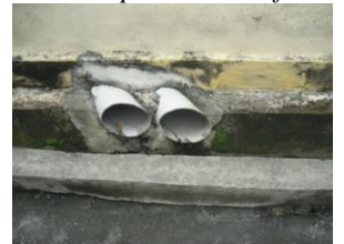
Specially built pipes to channel water away from flooding areas
