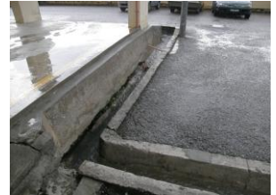
Sunken and cracked drains
